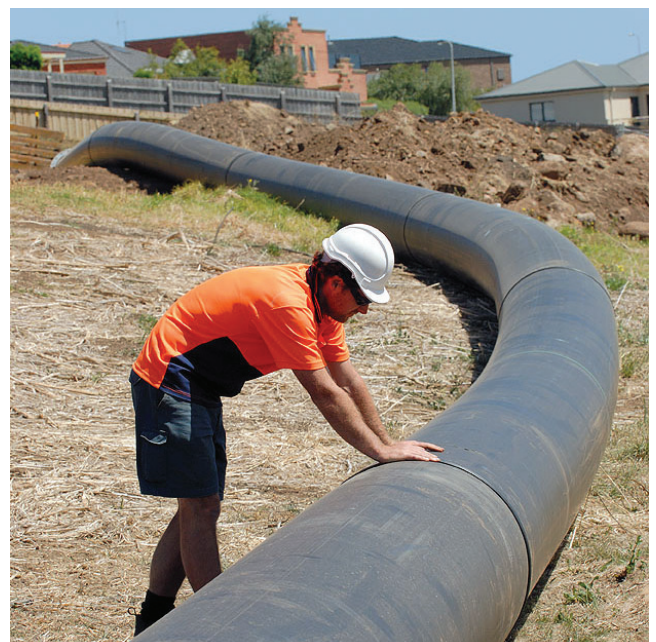
710mm polyethylene pipeline ready for laying to convey water (under pressure) from the subdivision to the storage basin.
