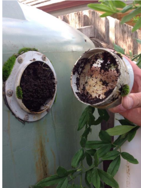
Figure 9: Fouled mosquito mesh at overflow which indicates high levels of sediment in the tank water.
