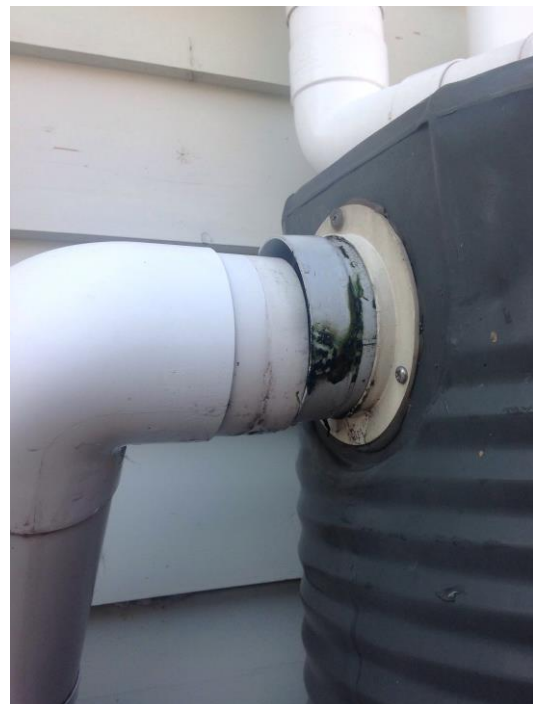
Figure 6: Fouling and leaking around overflow mesh. Disconnection indicates tank may have moved.
