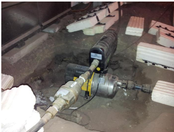
Figure 21: Equipment installed at a second study site
