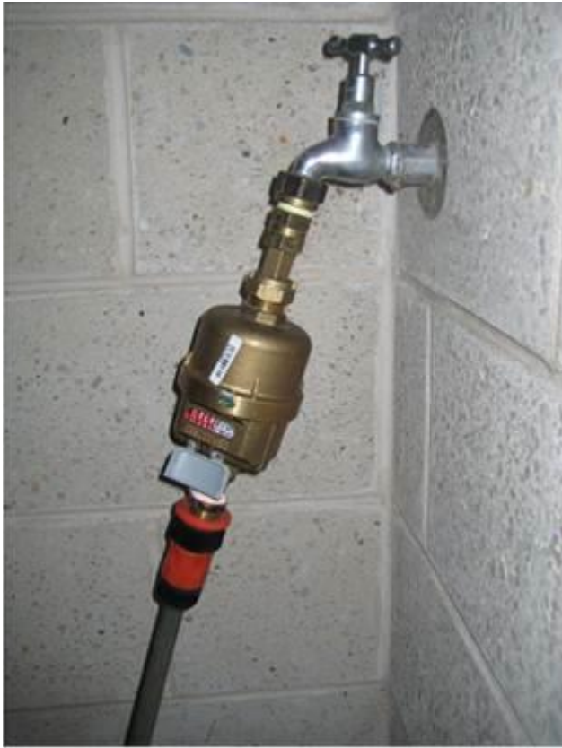
Figure 24: Flow meter connected to garden tap
