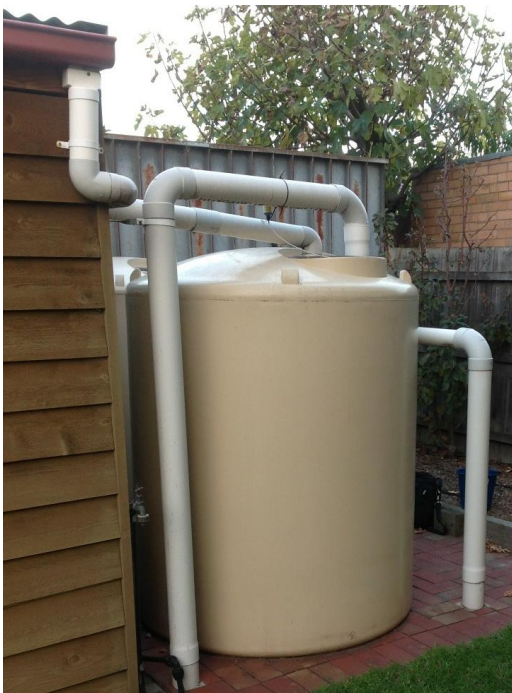
Figure 4: Polycarbonate tank with direct downpipe inflow and wet charge system. Tank installed on pre-existing paving.
