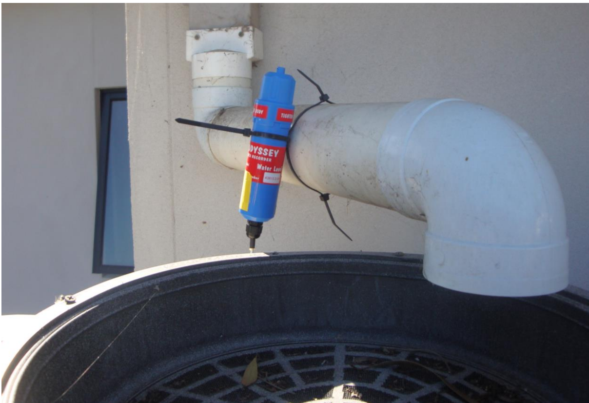
Figure 25: Depth gauge connected to tank
