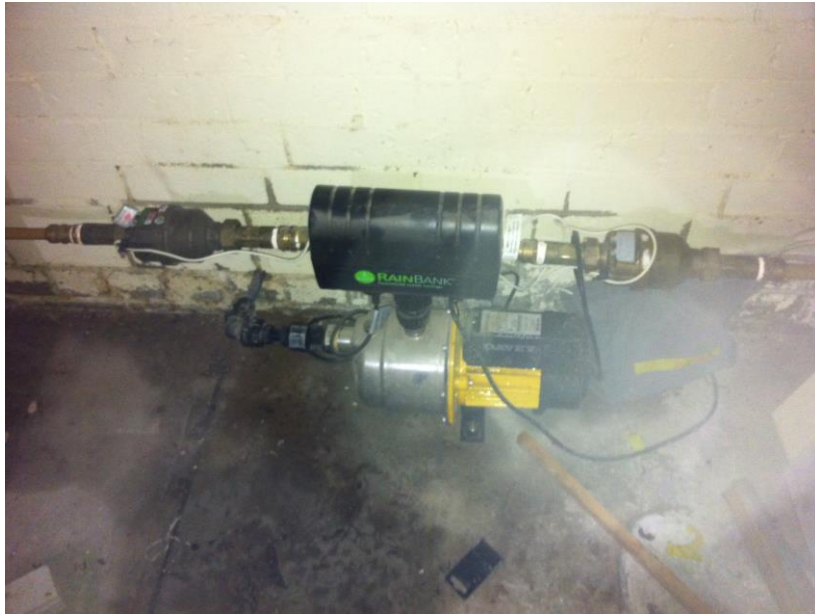
Figure 22: Photo of a pump with meters
