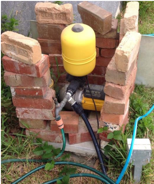
Figure 12: Pump with pressure vessel.
