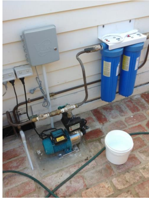
Figure 13: Pump system with copper piping and dual filters (pump enclosure not visible).
