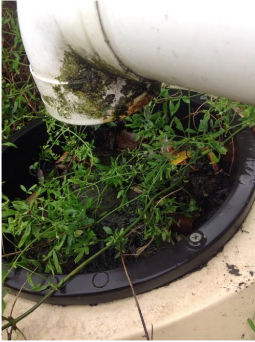
Figure 7: Inlet filter full of debris and vegetation.
