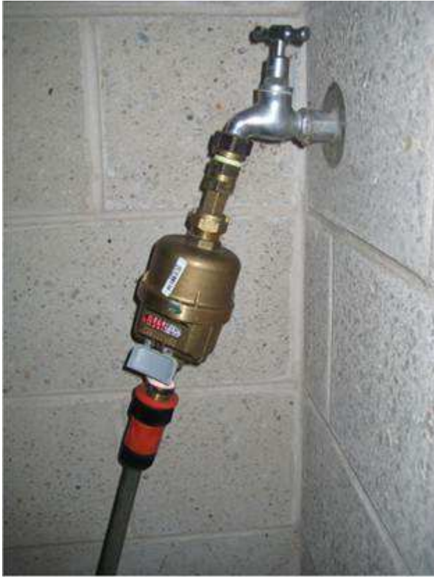
Figure 24: Flow meter connected to garden tap
