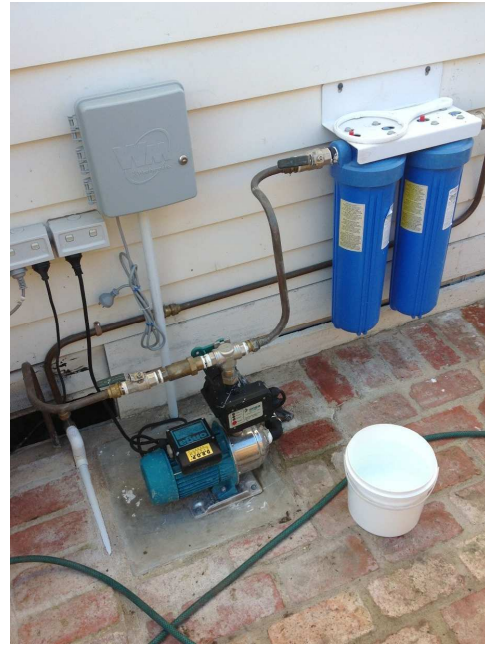
Figure 13: Pump system with copper piping and dual filters (pump enclosure not visible).
