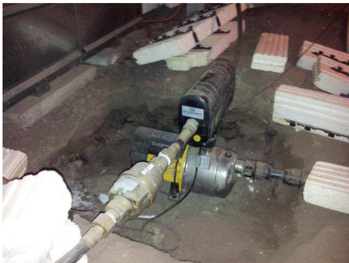
Figure 21: Equipment installed at a second study site
