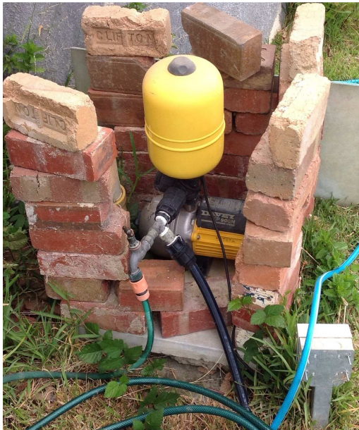
Figure 12: Pump with pressure vessel.
