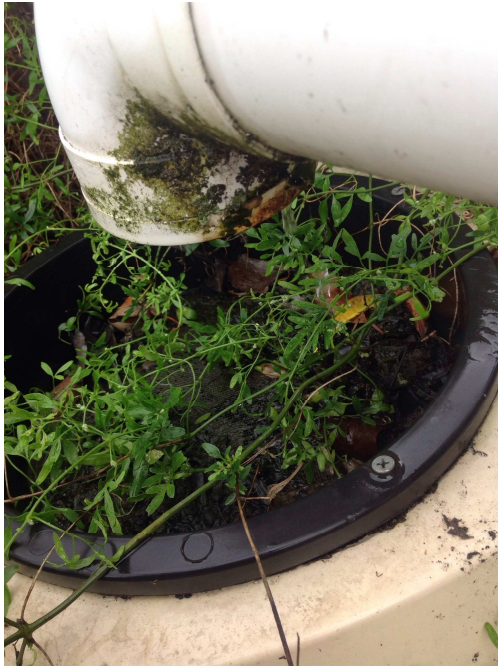
Figure 7: Inlet filter full of debris and vegetation.
