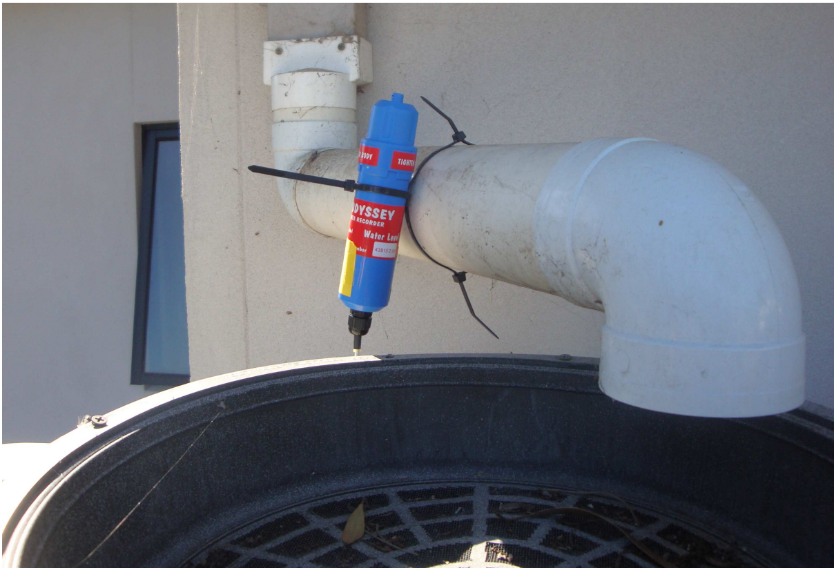
Figure 25: Depth gauge connected to tank
