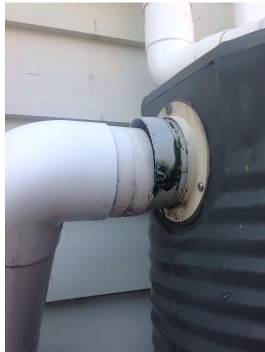
Figure 6: Fouling and leaking around overflow mesh. Disconnection indicates tank may have moved.
