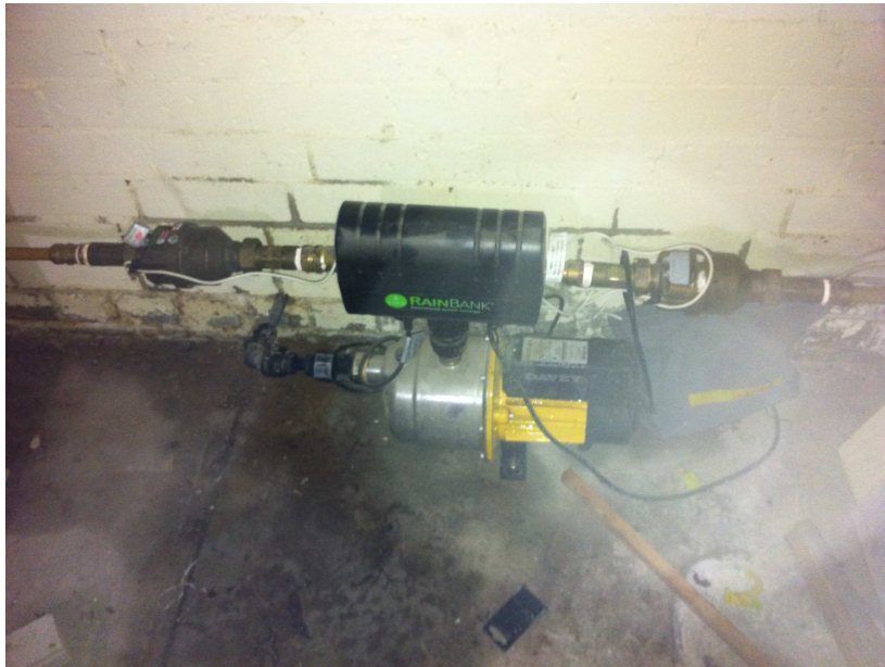
Figure 22: Photo of a pump with meters
