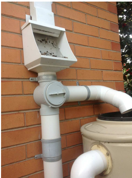
Figure 8: Rain-head and stormwater switch installed prior to tank inlet.
