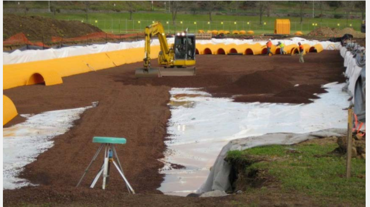
The additional storage tank built in 2008 is located under a sports field (Photo courtesy of City of Melbourne)
