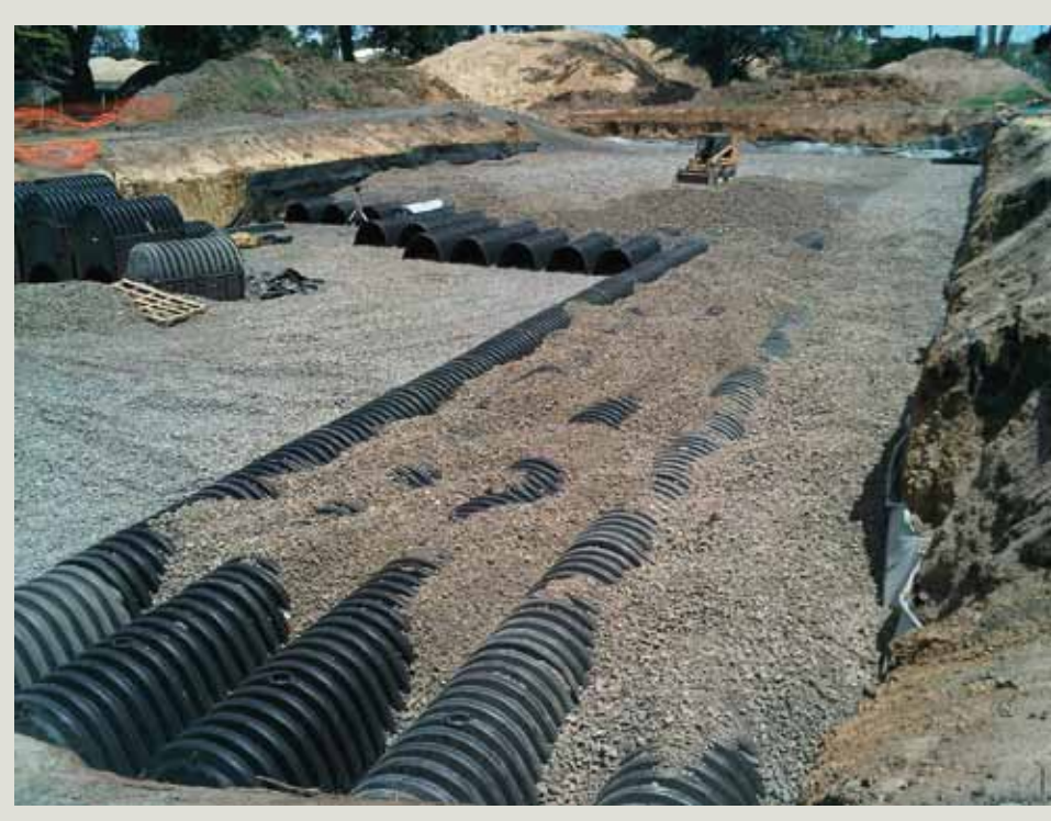
1km of plastic chambers are buried in 4000 tonne of rock encased in a high density plastic liner
